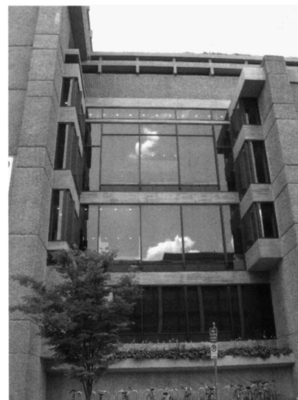
Fig. 6. Installation of new insulating glazing at the east facade, Paul Rudolph Hall, photograph 2008. Courtesy of Hoffmann Architects, Inc.
