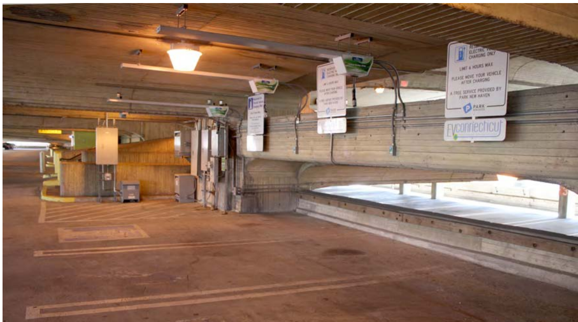
Photo 15. Interior view of upper level showing new electric vehicle charging stations, camera facing north.
