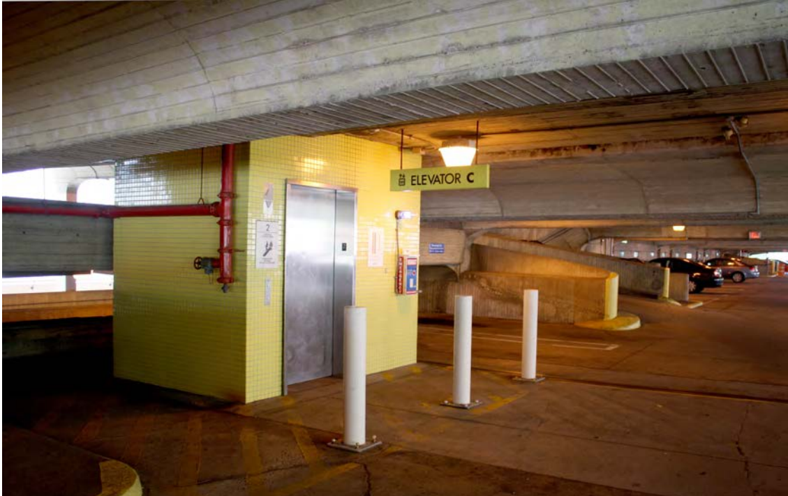
Photo 14. Interior view of upper level showing (south) yellow elevator bank, camera facing southeast.
