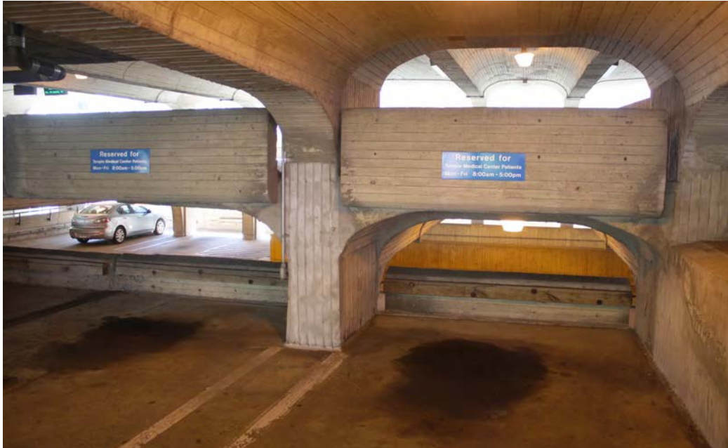
Photo 16. Interior upper level view (south of George Street) of typical structural bays including the central north-south line of piers with integral guard walls and the staggered floor levels with paired transverse beams. Camera facing east.
