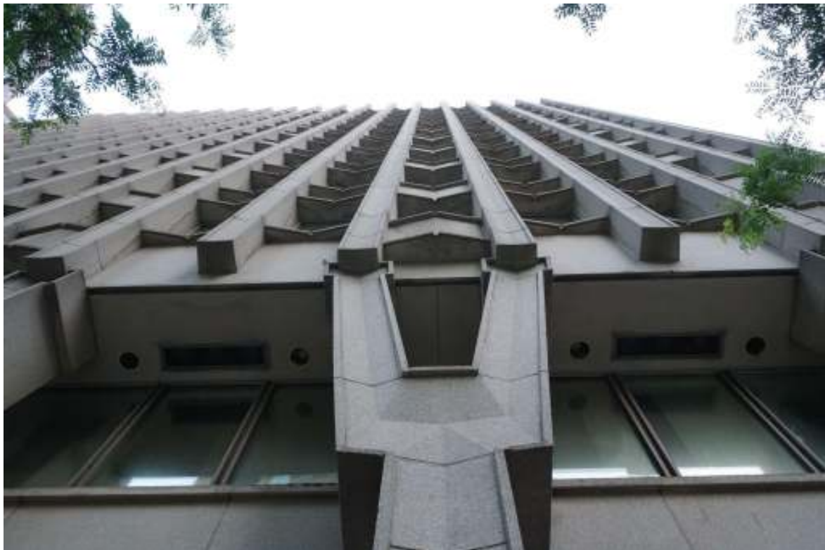
Figure 7. View from below south elevation showing Y-shaped columns, V-cutouts in sills, and concrete columns rising to the cornice, June 2023. Photo credit: Building Conservation Associates.
